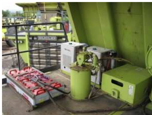
The Cells (2x) Installed on the massive deck of this Truck
